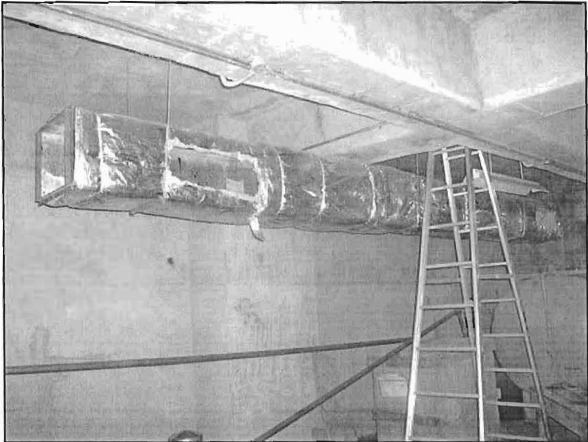
Power House Ventilation Duct
