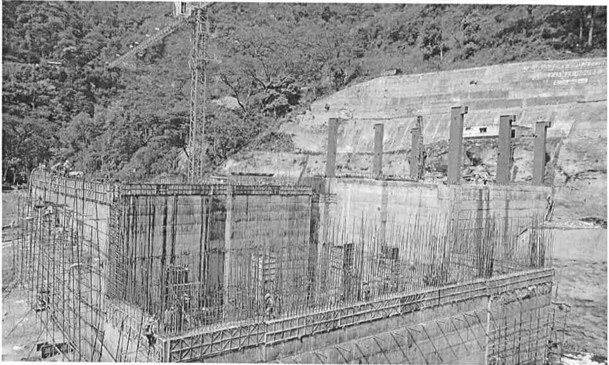
View of Power House-Concreting, reinforcement binding, shuttering and structural steel erection work under progress
